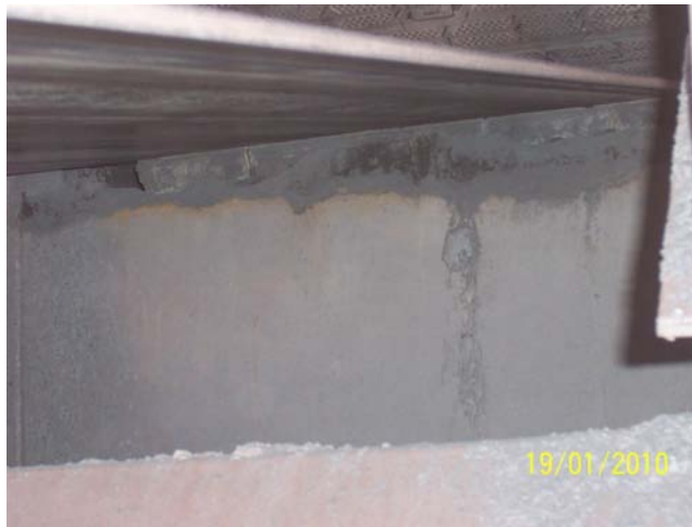
Photo 2 (Material build-up on frame near pulley.)
