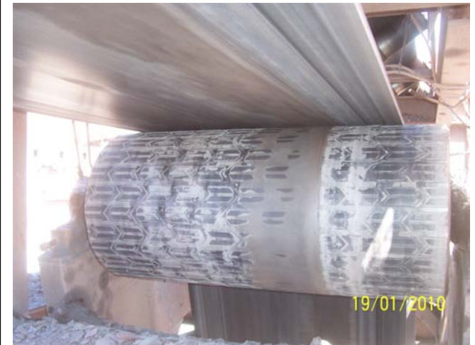
Photo 3 (Material build-up on lagging tread at center.)
