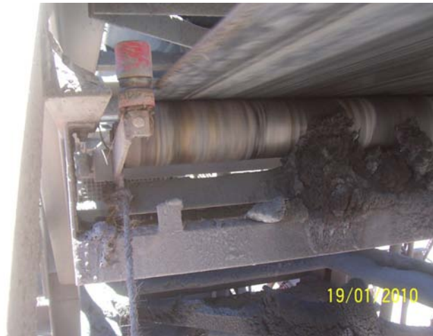
Photo 2 (Frame does not freely rotate and excess material build-up.)
