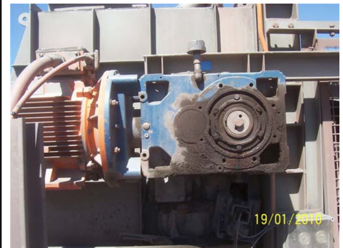
Photo 6 (No cover to open ended shaft of motor gearbox.)
