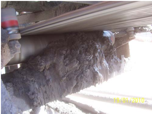
Photo 1 (Excess material build-up around return idler.)
