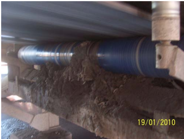
Photo 1 (Frame does not freely rotate and excess material build-up.)
