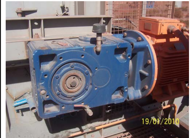
Photo 3 (No cover to open ended shaft of motor gearbox.)
