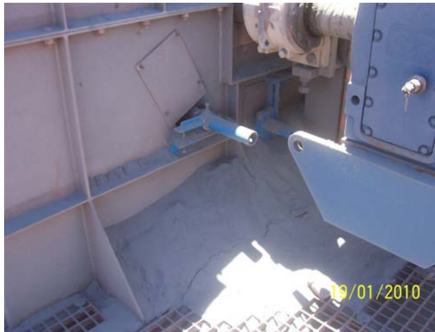
Photo 2 (Signs of material build-up near head end cleaners.)
