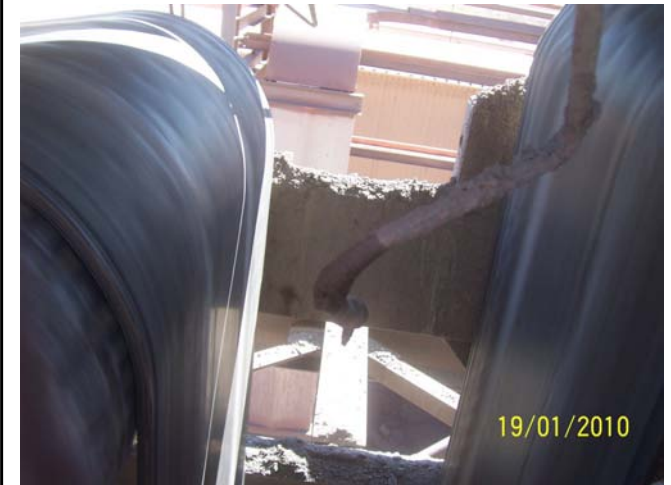
Photo 3 (Lube line bent and not connected at TS TUP pulley.)
