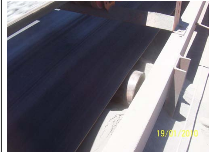
Photo 3 (Excessive material build-up near tru-tracker frame # 142.)
