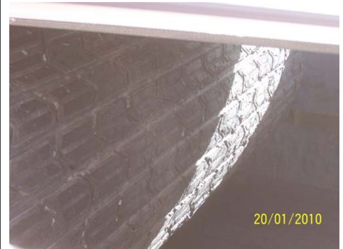
Photo 6 (Cracking and gouges to pulley lagging at center.)
