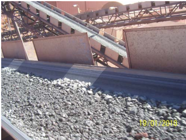
Photo 1 (Section 3m long on LHS edge torn back to carcass.)
