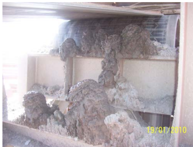
Photo 5 (Excess material build-up on frame near TS TUP.)
