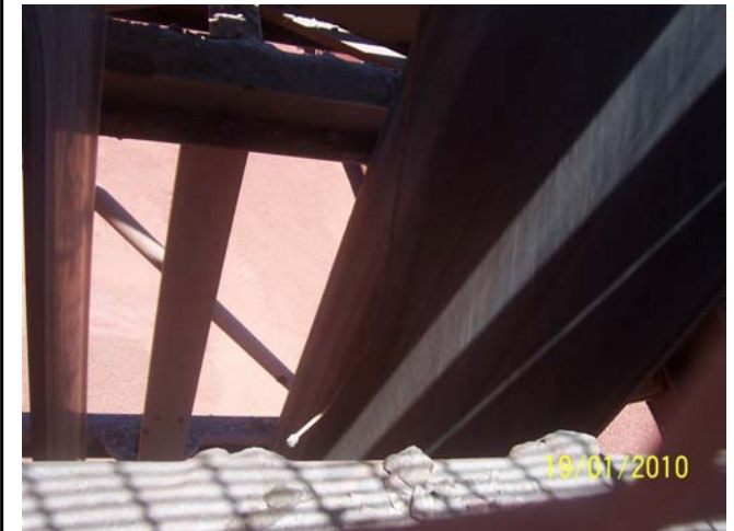
Photo 3 (Lube line limited access head side TUP bend pulley.)
