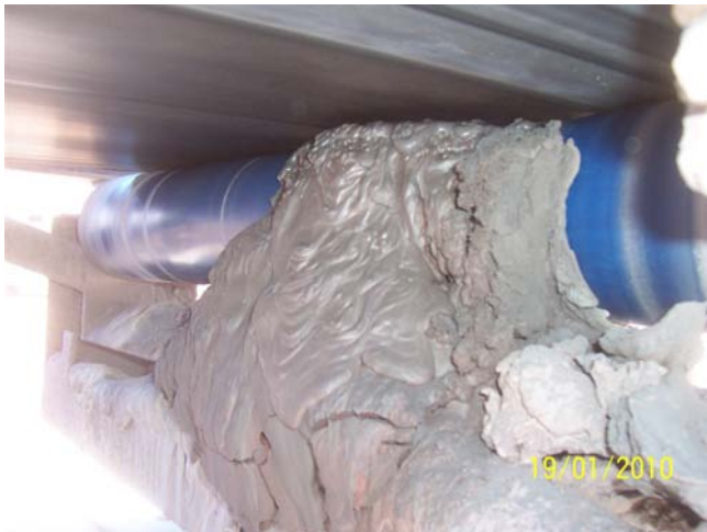
Photo 1 (Excess material build-up around tracking idler.)
