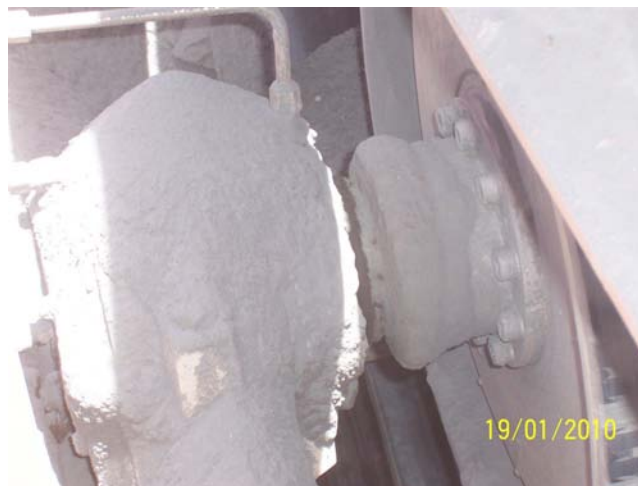
Photo 5 (Grease & dust build up on LHS pulley shaft.)
