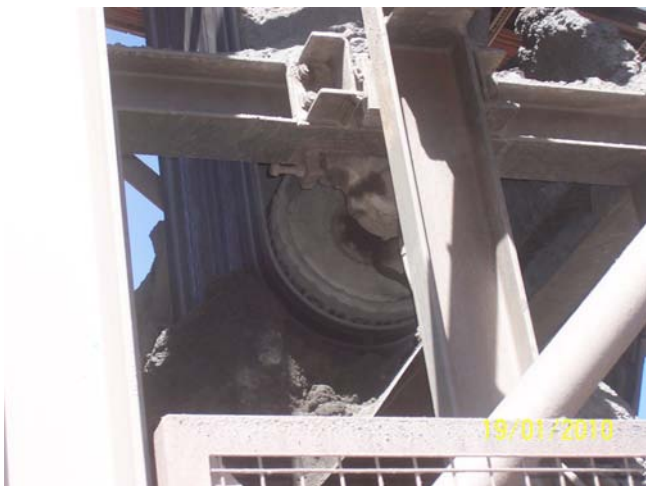
Photo 4 (Material build-up around TUP pulley.)
