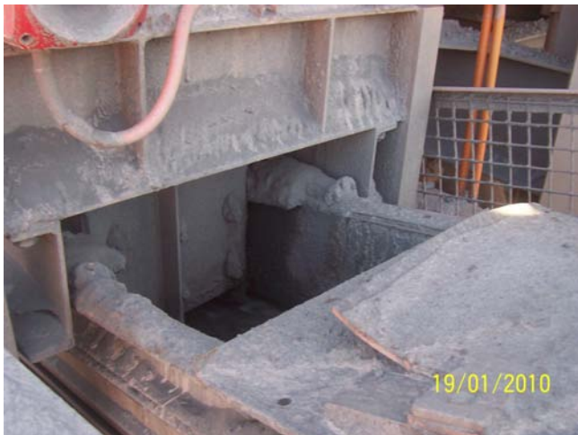
Photo 4 (Chute cover at tail end transfer requires readjusting.)
