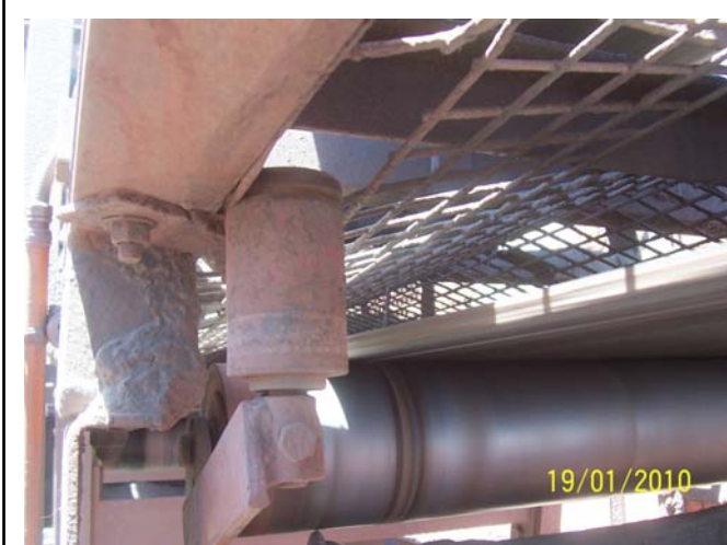
Photo 1 (RHS servo of return tracker hitting structure.)
