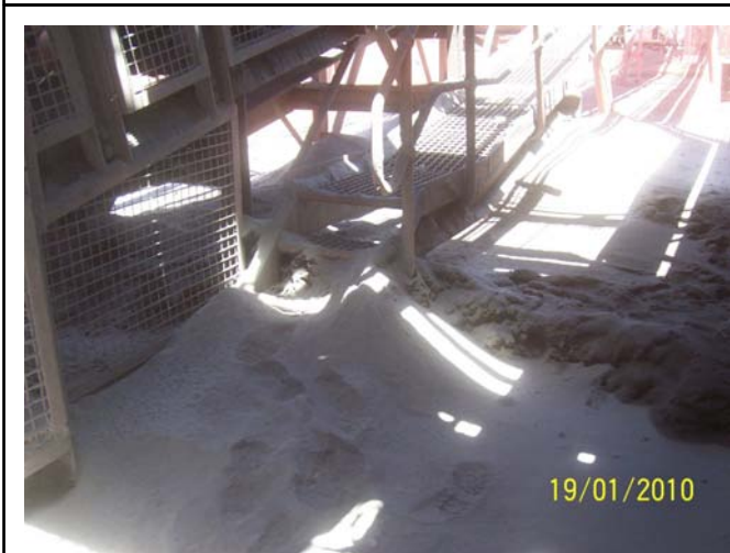
Photo 4 (Excess material build-up at tail end of conveyor.)
