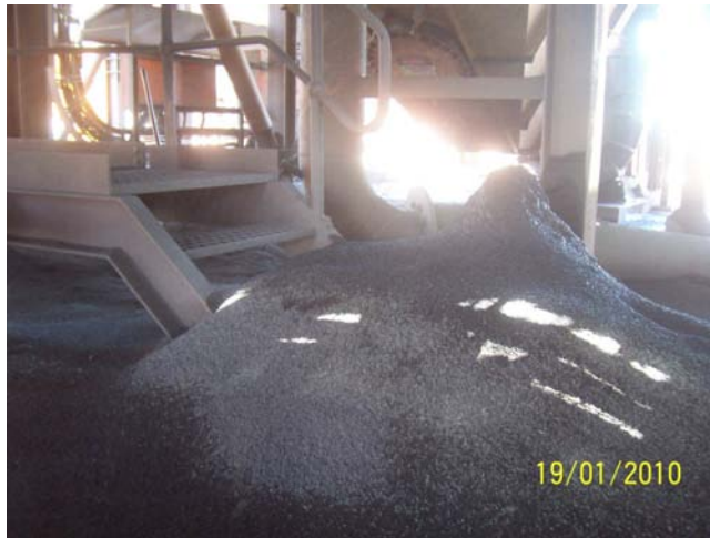
Photo 8 (Excess material build-up at tail end LHS/RHS walkways.)
