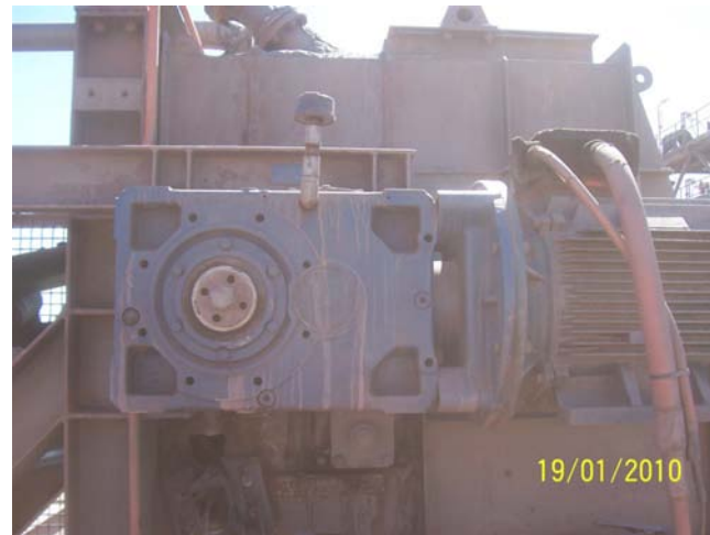
Photo 2 (No cover to open ended shaft of motor gearbox.)
