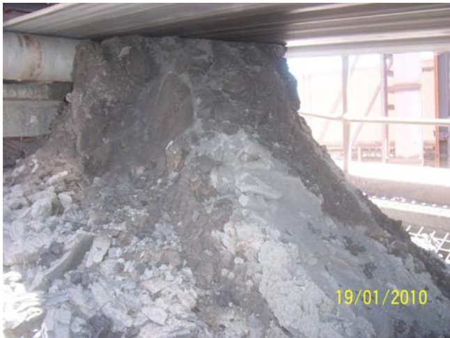
Photo 7 ( Excess material build-up around return idlers from Tail onwards.)
